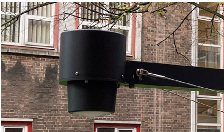
Figure 40. Radar sensor with protective cover.
