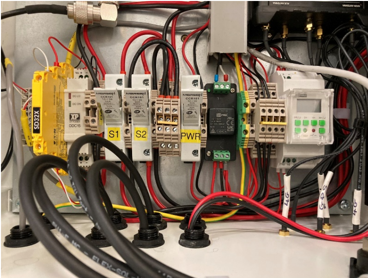
Figure 27. Logger switched fuses in the open position.
