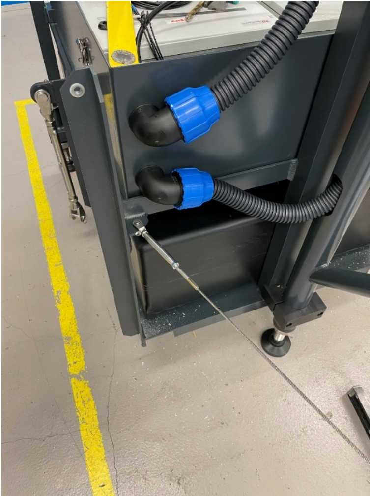
Figure 12. Guy wire attached to main frame with turnbuckle adjustment.
