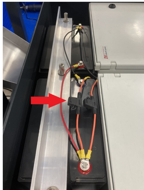
Figure 21. Batteries installed in parallel configuration. Mini blade fuse holders are indicated by the red arrow.
