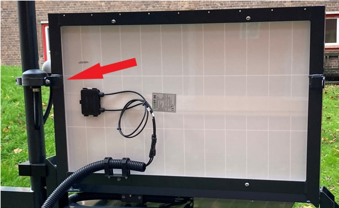
Figure 17. Solar panels locked in place.
