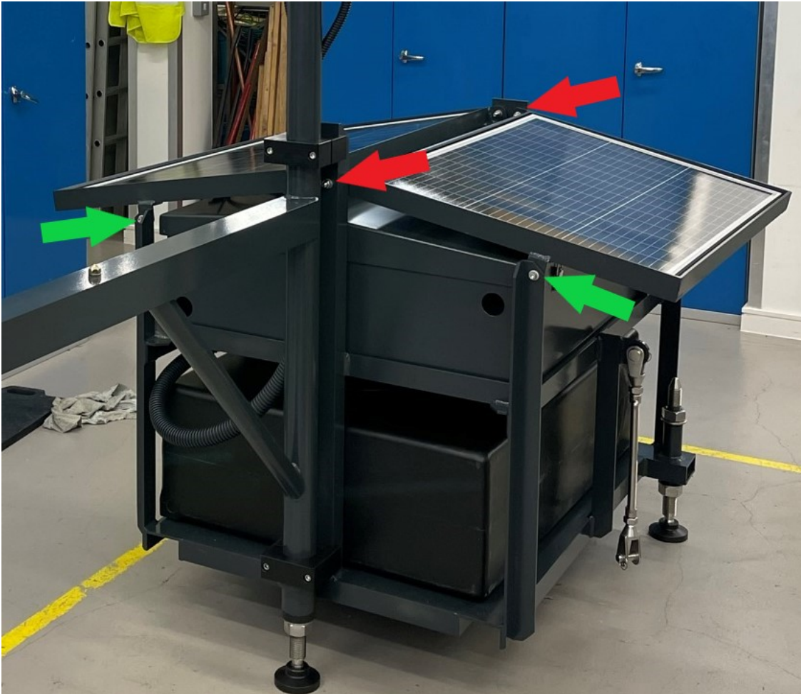
Figure 16. Solar panel mounting bolt locations. Green arrows indicate bolts removed for accessing equipment enclosures.
